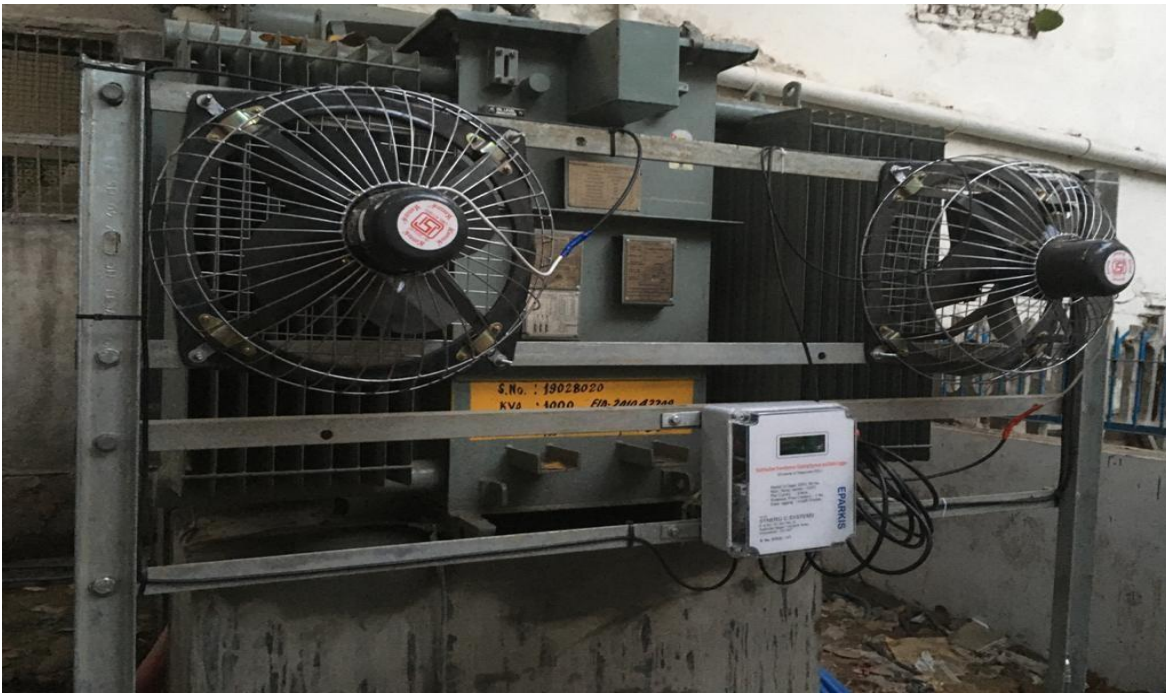
Plinth mounted DT with auto cooling system
